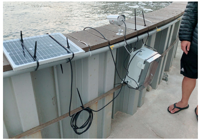
Figure 4. IoT monitoring system
